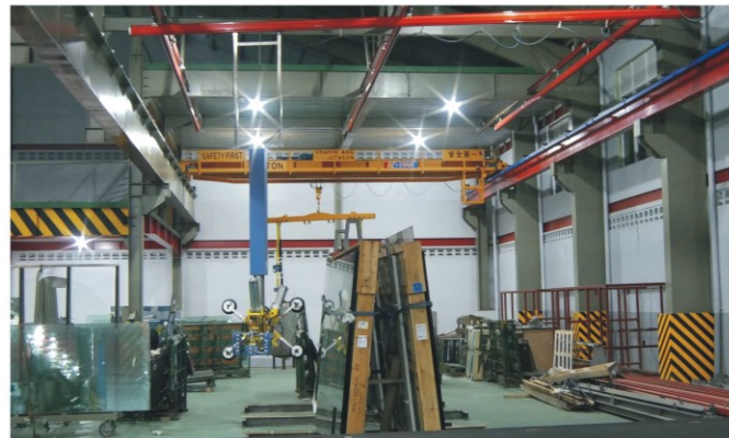
Overhead crane with LRS system
